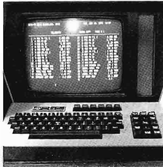
Keyboard and CRT display unit for DCS-2 system located in the transmitter control area.
