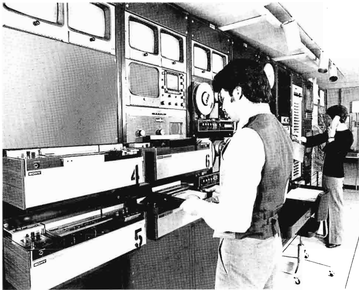
"House" TV distribution system permits sending up to eight video programs simultaneously to 150 locations throughout Merrill Lynch headquarters.
